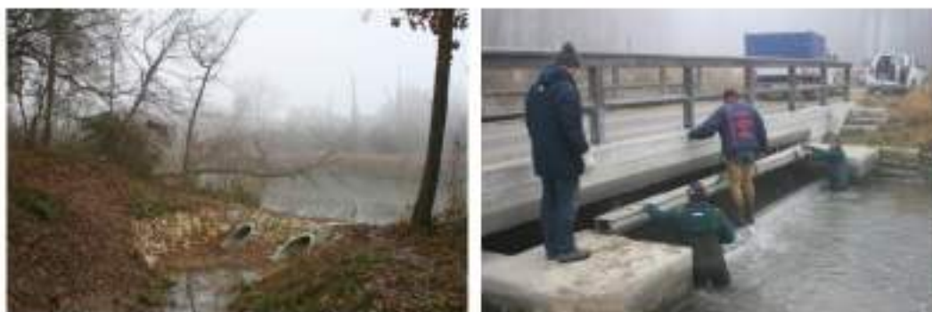
Figure 18: Structures for groundwater lowering. Left: Diversion structure from the "Old Danube" to the diversion channel. Right: Insertion of the dam beams by WWA Ingolstadt into the 2nd cut-off structure (Photos: Peter Fischer)
